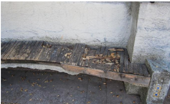
Linear Park Oak Glen Bench in Need of Repair
