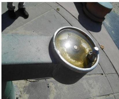
South Prescott—Plugged fountain
