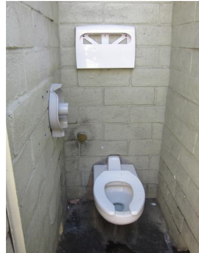
The Women’s restroom at Lowell was clean but missing toilet paper.
