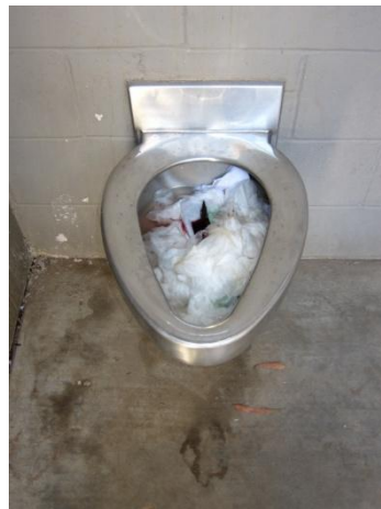
North Oakland Regional Sports Center—clogged toilet
